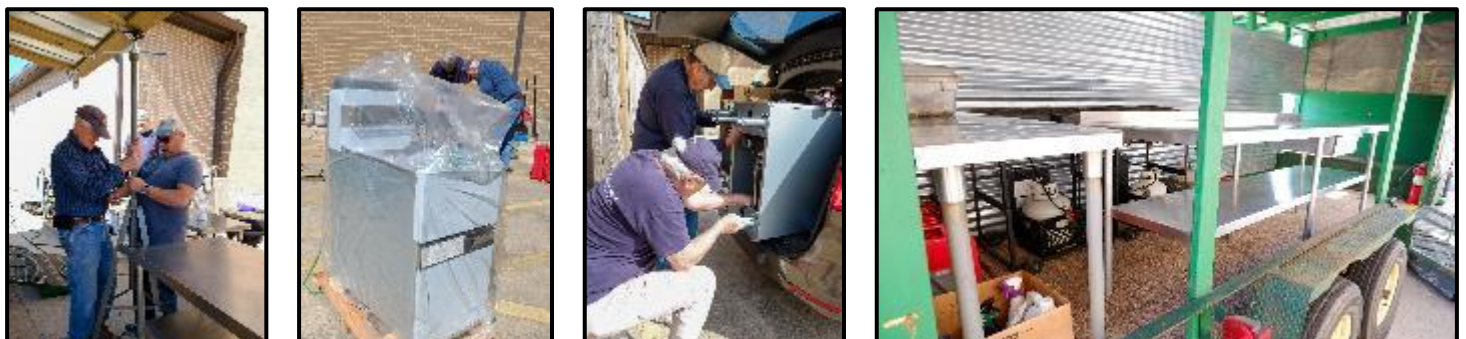
Positioning safety stand; one of the new fryers; putting legs on a new fryer; a clean trailer
